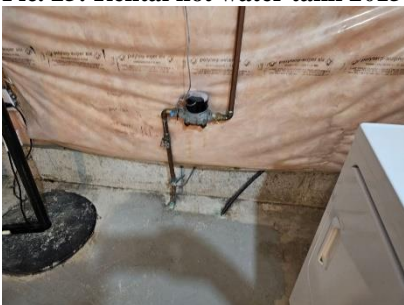
Pic. 28: Water main
