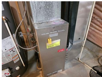
Pic. 26: Gas furnace 1997
