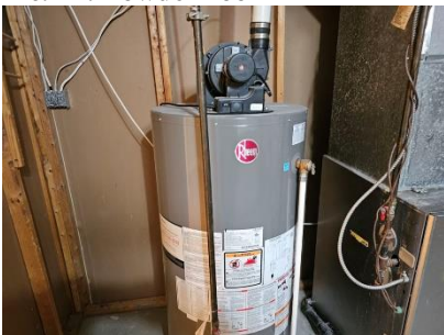
Pic. 25: Rental hot water tank 2015
