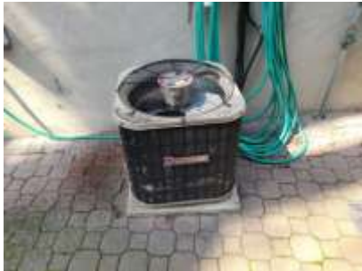
Pic. 4: AC unit 1984
