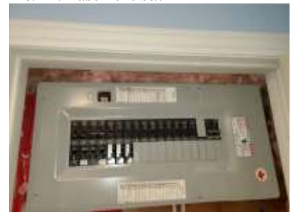
Pic. 27: 100 amp breaker panel
