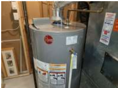
Pic. 28: Rental hot water tank 2015
