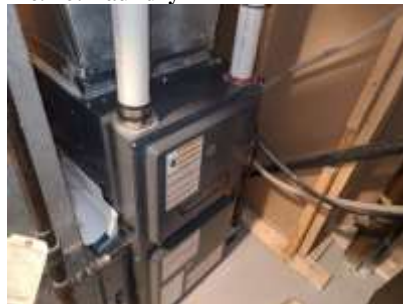
Pic. 29: Gas furnace 2016
