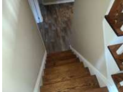
Pic. 20: No hand railing for basement stairwell
