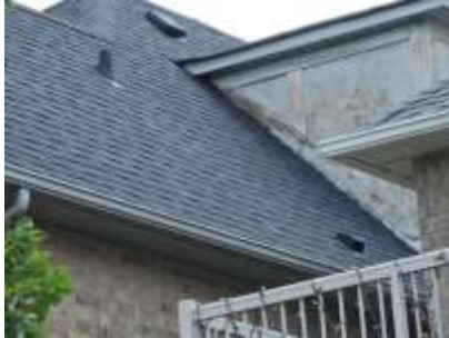
Pic. 4: Wood trim area could use painting maintenance
