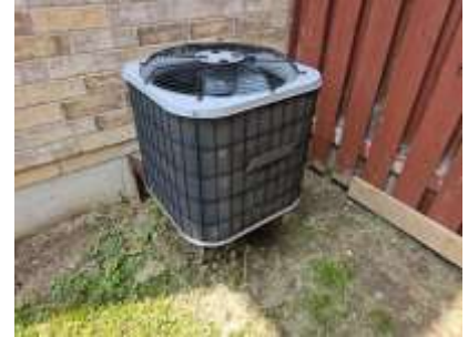
Pic. 6: AC unit 2004
