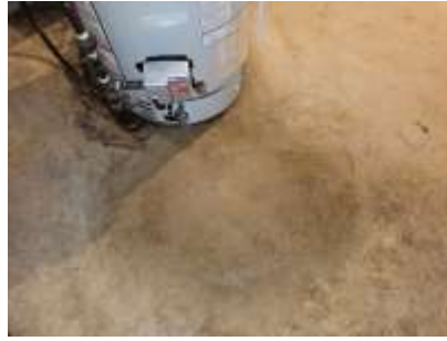
Pic. 32: Puddle on floor at hot water tank recommend have the tank reviewed
