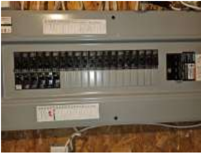
Pic. 34: 200 amp breaker panel
