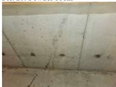
Pic. 29: Foundation crack with a visible repair on the exterior of the home
