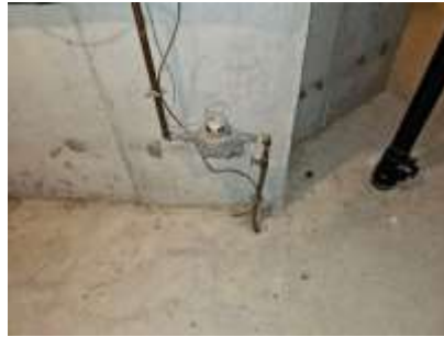
Pic. 35: Water main
