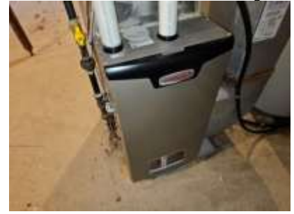
Pic. 33: Gas furnace 2020
