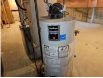
Pic. 31: Hot water tank 2020
