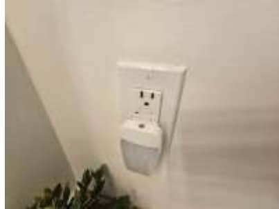
Pic. 17: Bathroom and powder room GFCI outlet defective
