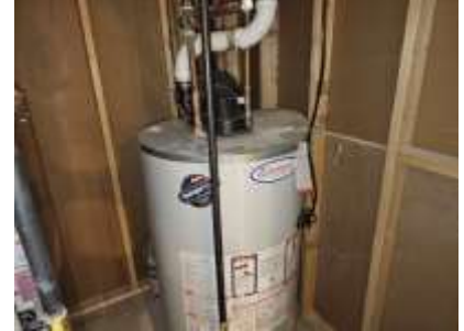
Pic. 33: Rental hot water tank 2023
