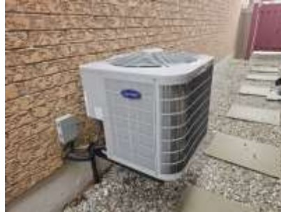
Pic. 5: AC unit 2022
