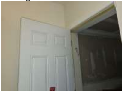
Pic. 10: No auto closer on garage entry door
