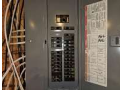
Pic. 35: 100 amp breaker panel
