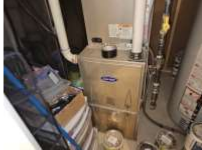
Pic. 32: Gas furnace 2022
