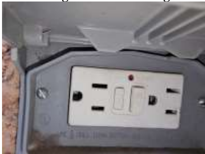
Pic. 7: Exterior GFCI outlets not working
