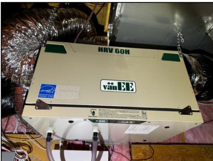
15. Heat recovery ventilator (HRV)
