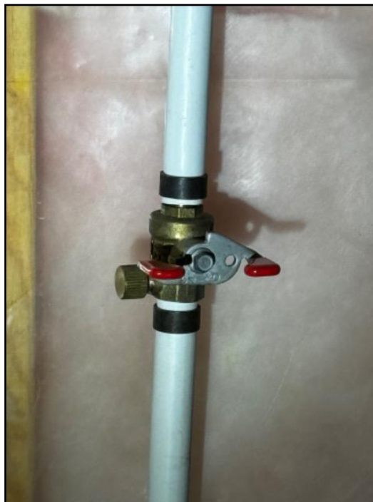
24. Hosebib shut off valve
