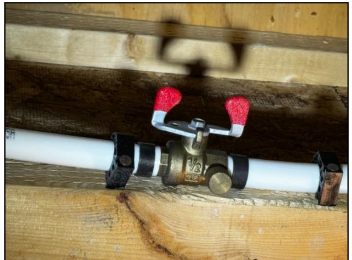
23. Hosebib shut off valve
