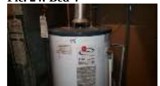
Pic. 28: Rental hot water tank
