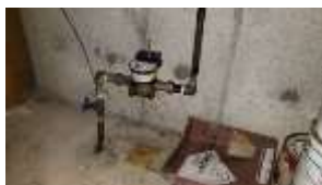
Pic. 30: Water main
