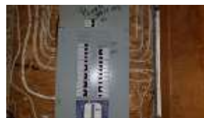
Pic. 31: : 100 amp breaker panel
