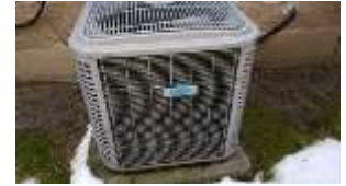
Pic. 4: AC unit 2017
