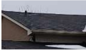
Pic. 2: Missing shingle tab above the plumbing stack pipe
