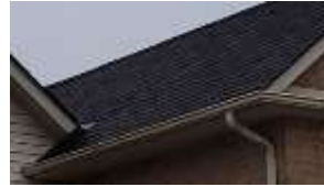
Pic. 3: Roof covering is aging
