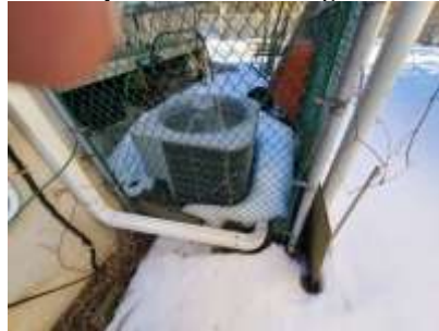
Pic. 5: AC unit 2014
