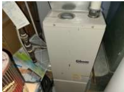
Pic. 26: Gas furnace 2009
