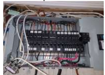
Pic. 27: 100 amp breaker panel
