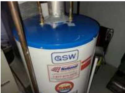
Pic. 25: Rental hot water tank
