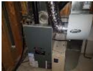
Pic. 34: High efficiency gas furnace
