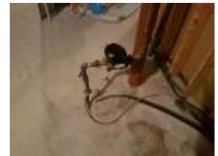
Pic. 36: Water main
