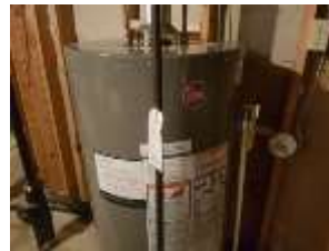
Pic. 35: Rental hot water tank
