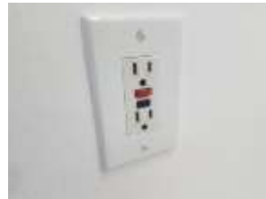
Pic. 15: Defective GFCI
