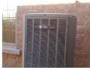
Pic. 6: AC unit 2003
