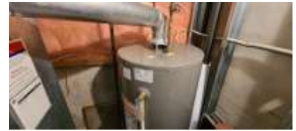
Pic. 33: Rental hot water tank 2013
