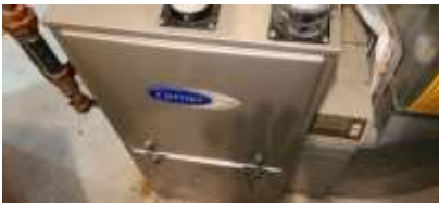
Pic. 34: Gas furnace 2014
