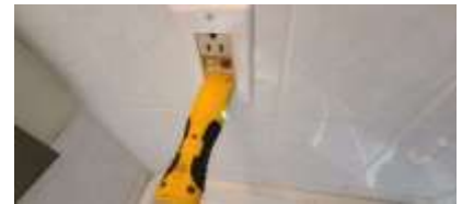
Pic. 27: GFCI outlet in powder room won't trip
