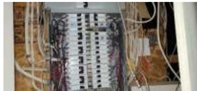
Pic. 35: 100-amp breaker panel
