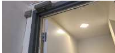
Pic. 8: Garage entry door auto closr disconnected
