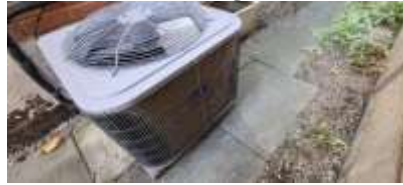
Pic. 5: AC unit 2018
