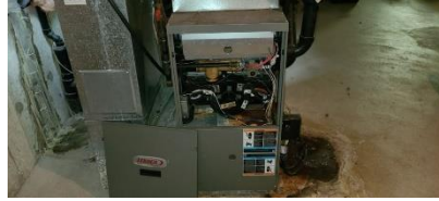
Pic. 44: Gas furnace 2006
