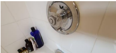
Pic. 25: Water diverter seized in the shower position
