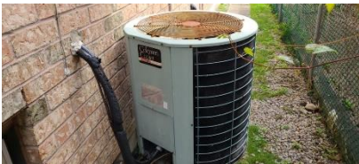
Pic. 7: Old AC compressor, budget for replacement
