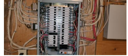
Pic. 45: 200-amp breaker panel
