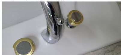
Pic. 17: Water diverter on tub is leaking
