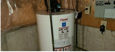
Pic. 43: Rental hot water tank 2022
