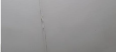
Pic. 28: Corner tapping lifting, does not appear to be from water leaking
