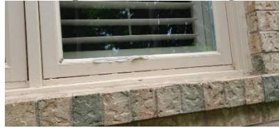
Pic. 5: Some of the wooden window frames in need of painting maintenance
