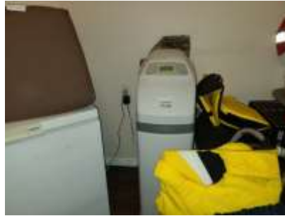
Pic. 35: Water softener
