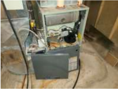
Pic. 34: Gas furnace 2011
