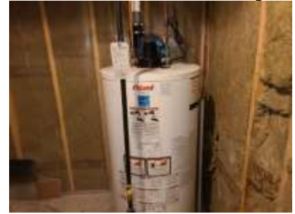
Pic. 33: Rental hot water tank
