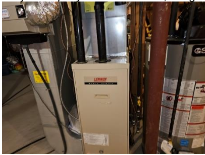
Pic. 31: Original gas furnace
