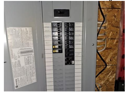
Pic. 33: 200 amp breaker panel
