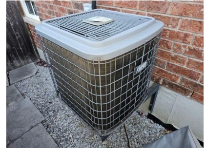
Pic. 6: Original AC unit
