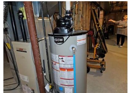
Pic. 30: Rental hot water tank 2019
