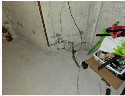
Pic. 32: Water main
