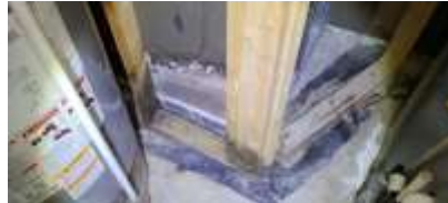
Pic. 11: Old water damage in utility room
