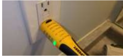
Pic. 23: GFCI outlet won't trip and need to be replaced – this outlet protects all three bathrooms
