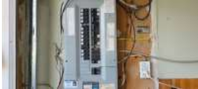
Pic. 7: 100 amp electrical panel
