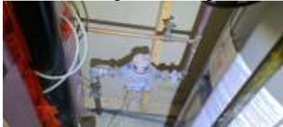
Pic. 10: Water main
