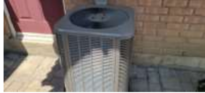
Pic. 5: AC unit 2017
