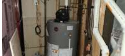
Pic. 8: Water heater 2017
