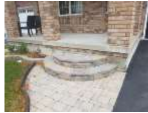
Pic. 3: Front steps with uneven rise
