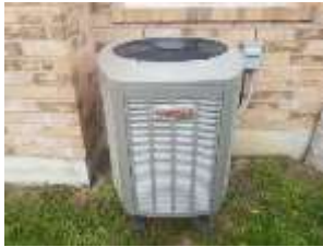
Pic. 5: AC unit 2016
