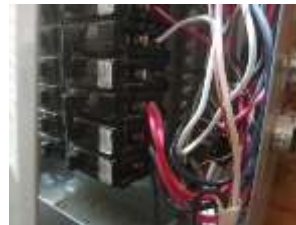
Pic. 39: 40 amp breaker for stove double tapped with dryer, needs immediately repair / correction
