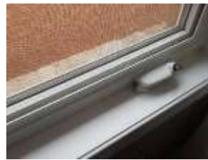
Pic. 15: Window crank in need of adjusting / repair
