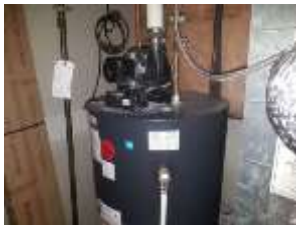
Pic. 37: Rental hot water tank
