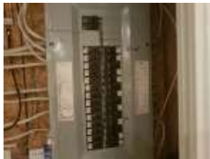
Pic. 38: 100 amp breaker panel with all copper wire
