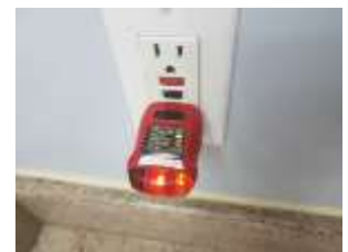
Pic. 20: Bath GFCI needs repair / replacement
