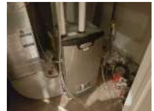
Pic. 36: High efficiency gas furnace 2016
