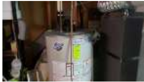
Pic. 42: Rental hot water tank 2018
