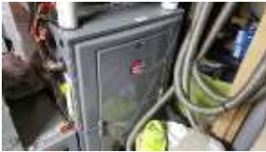
Pic. 41: Gas furnace 2018
