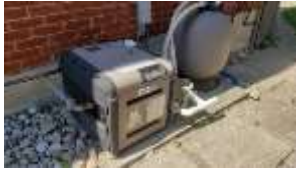
Pic. 5: Pool heater and pump equipment
