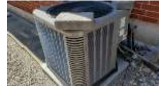
Pic. 4: AC unit 2018
