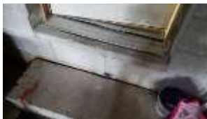
Pic. 13: An additional step advised at garage entry door
