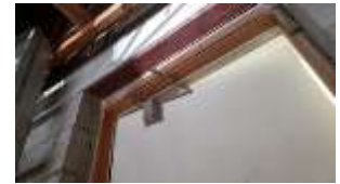
Pic. 12: Auto closer disconnected
