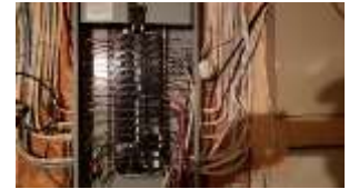
Pic. 44: 100 amp amin breaker panel. A couple of breakers are double tapped
