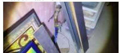
Pic. 39: Water main
