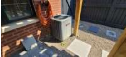
Pic. 7: AC unit #2 2017
