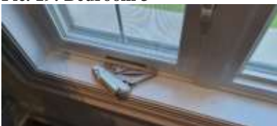
Pic. 22: Broken window crank
