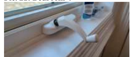
Pic. 24: Broken window crank
