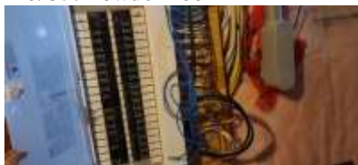
Pic. 38: 200 amp breaker panel
