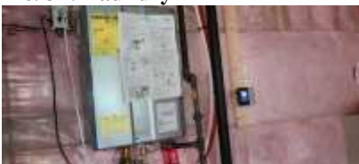
Pic. 37: Tankless hot water system
