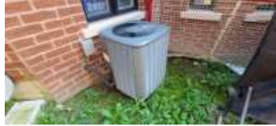
Pic. 5: AC unit #1 2017
