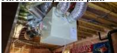
Pic. 41: HRV system
