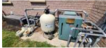
Pic. 5: Pool equipment
