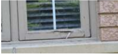
Pic. 4: Some rot to window frames
