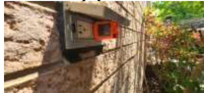
Pic. 8: Rear GFCI won't trip
