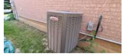
Pic. 3: Ac unit 2015
