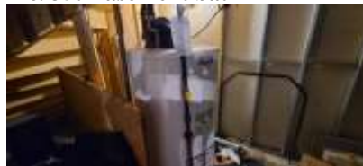
Pic. 38: Hot water tank 2018
