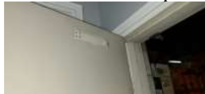
Pic. 11: Missing garage entry door auto closer
