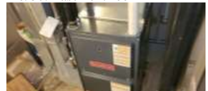
Pic. 39: Gas furnace 2020
