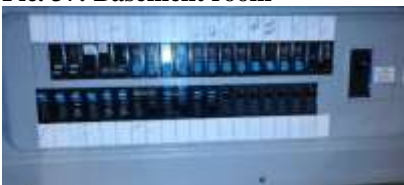
Pic. 40: 200 amp main breaker panel
