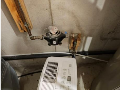
Pic. 34: Water main
