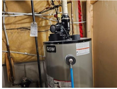
Pic. 32: Rental hot water tank 2017
