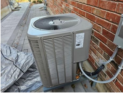
Pic. 4: AC unit 2020
