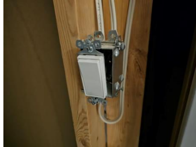
Pic. 35: Light switch in utility room needs to be properly secured
