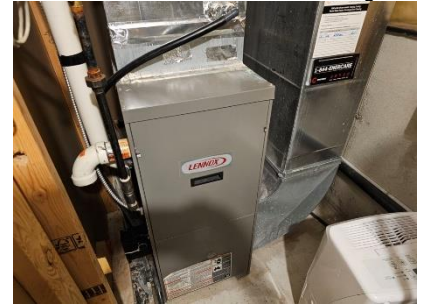
Pic. 33: Gas furnace 2008
