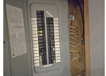
Pic. 36: 100 amp breaker panel
