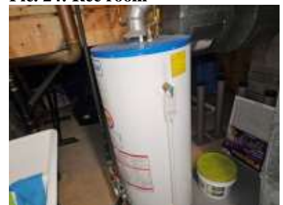
Pic. 27: Rebtal hot watert tank
