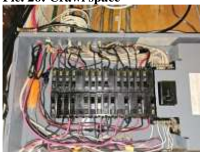
Pic. 29: 100 amp breaker panel
