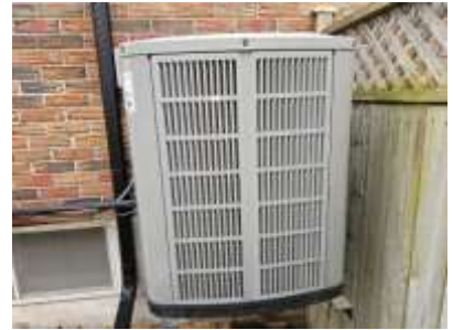
Pic. 6: AC unit
