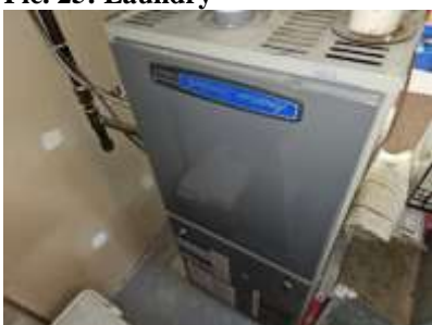
Pic. 28: Gas furnace
