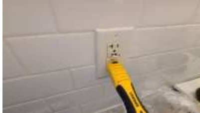
Pic. 23: Kitchen GFCI outlet reset button broken
