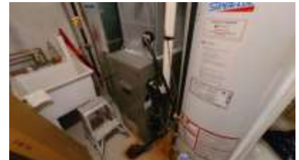
Pic. 33: Gas furnace 2008
