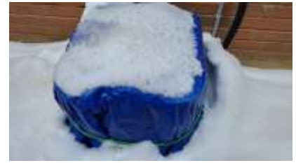
Pic. 3: AC unit
