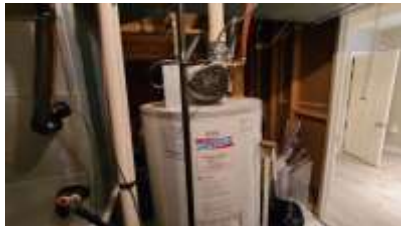
Pic. 32: Rental hot water tank 2008
