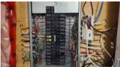
Pic. 34: 100 amp breaker panel
