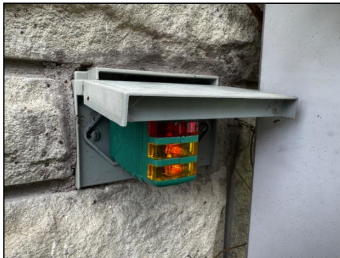
17. Test faulty on GFCI/GFI (Ground Fault...
