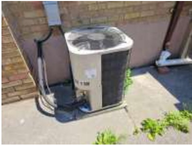
Pic. 4: AC unit 2008
