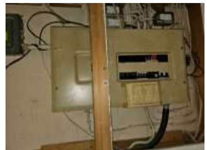
Pic. 27: 200 amp breaker panel
