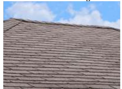
Pic. 9: Garage roof covering aging
