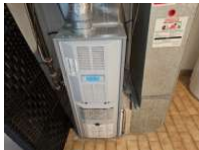
Pic. 26: Gas furnace 2007
