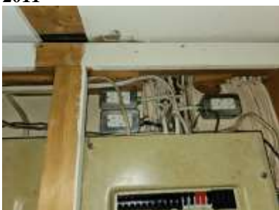
Pic. 28: GFCI protection for 2 wire ungrounded circuits
