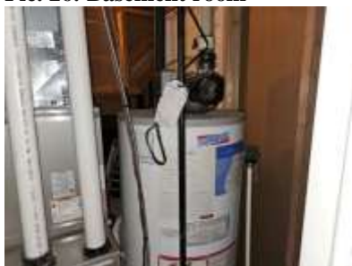
Pic. 29: Rental hot water tank 2010
