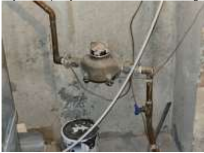
Pic. 31: Water main
