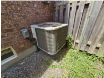
Pic. 4: AC unit 2018
