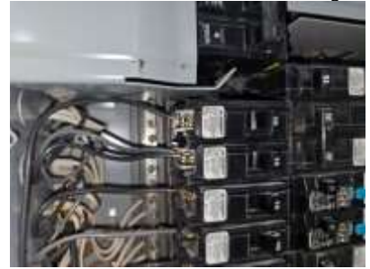
Pic. 33: Double tapped breaker
