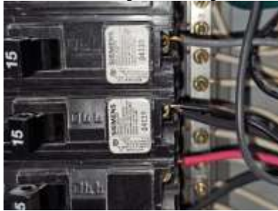
Pic. 35: Double tapped breaker
