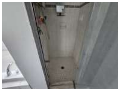
Pic. 14: Shower – water diverter seized
