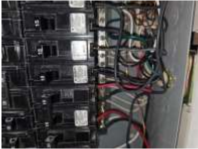
Pic. 34: Double tapped breaker
