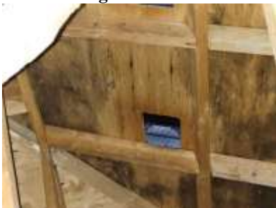
Pic. 10: Old staining – no active leaks
