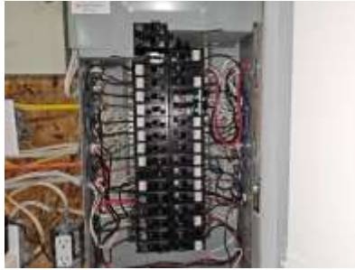
Pic. 32: 100 amp breaker panel
