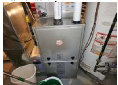
Pic. 30: Gas furnace 2018
