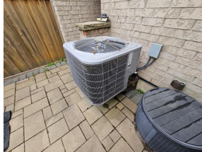
Pic. 5: AC unit 2013
