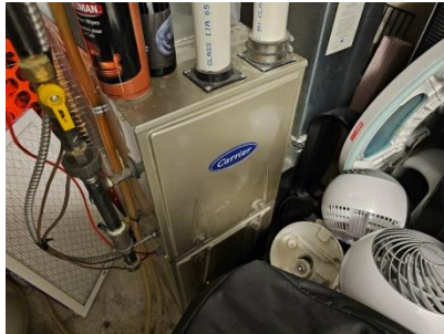
Pic. 26: Gas furnace
