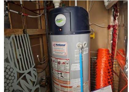
Pic. 24: Water heater
