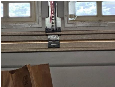
Pic. 7: Upper middle garage door hinged broken
