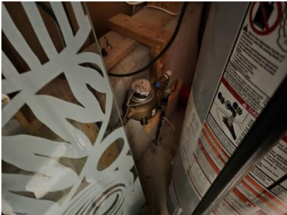
Pic. 25: Water main
