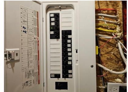
Pic. 27: 100 amp breaker panel
