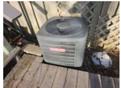
Pic. 12: AC compressor 2018
