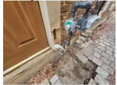
Pic. 6: Trim needs repair
