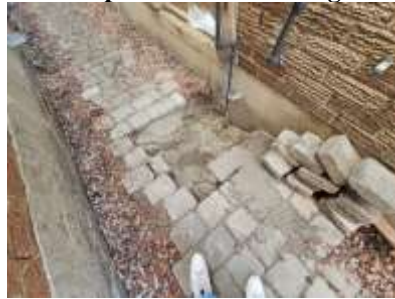
Pic. 5: Walkway needs repair
