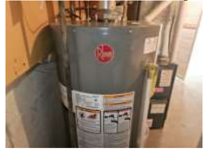
Pic. 33: Water heater 2025
