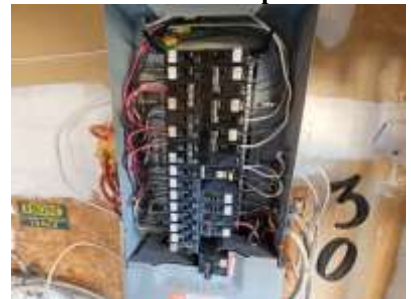
Pic. 9: 100 amp breaker panel
