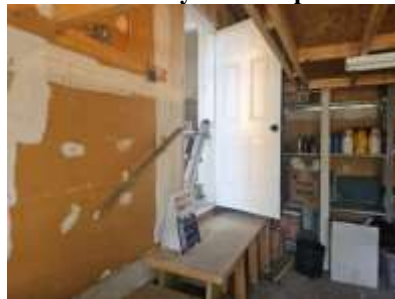
Pic. 8: Railing advised for entry landing in garage
