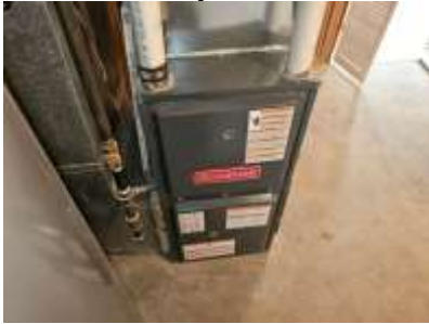
Pic. 34: Gas furnace 2019
