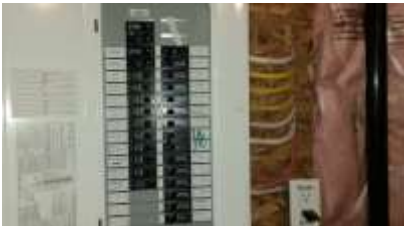
Pic. 31: 100 amp breaker panel
