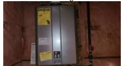
Pic. 30: Tankless hot water system 2018
