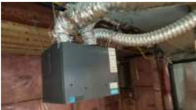
Pic. 28: HRV system
