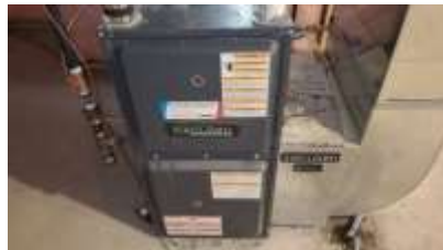
Pic. 29: Gas furnace 2018
