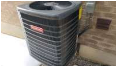
Pic. 4: AC unit 2017
