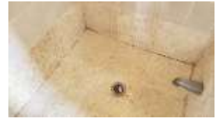
Pic. 12: Caulking needed in the shower
