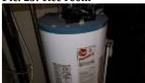
Pic. 29: Rental hot water tank
