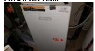
Pic. 28: Gas furnace 2002
