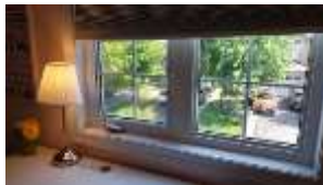
Pic. 14: Window cranks stripped
