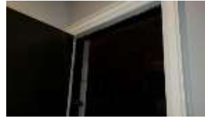
Pic. 19: Garage entry door – auto closer required
