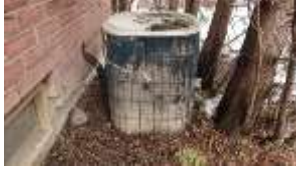
Pic. 5: Original AC in poor condition
