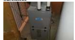
Pic. 32: Gas furnace 2017
