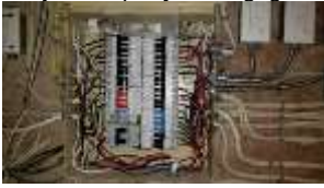
Pic. 33: 200 amp breaker panel
