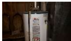
Pic. 31: Rental hot water tank
