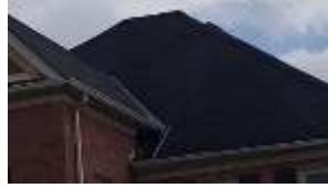
Pic. 2: Aging roof covering
