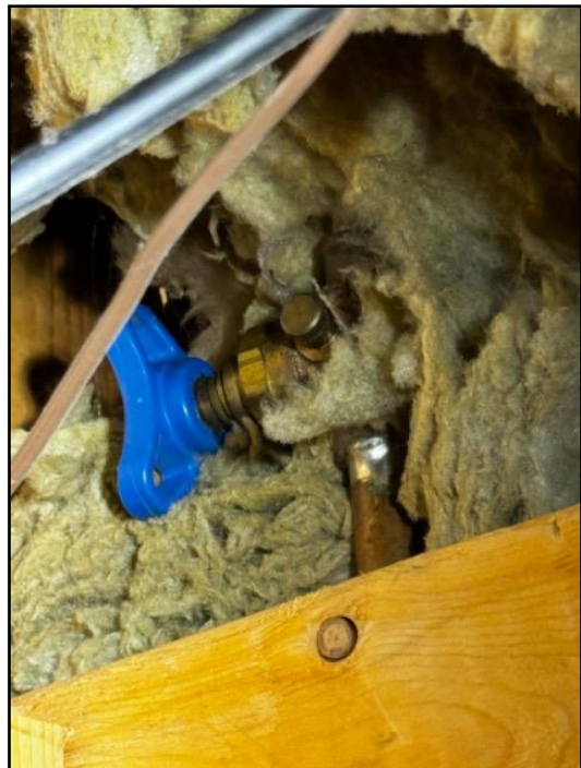
28. Hosebib shut off valve
