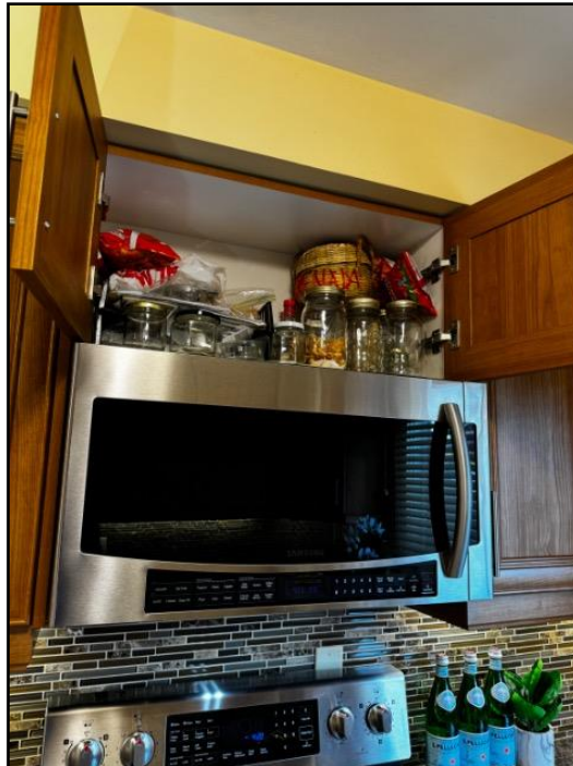
47. Not vented to exterior
