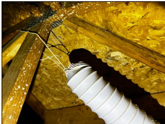
45. Does not discharge to exterior
