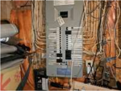
Pic. 46: 200 amp main breaker panel`
