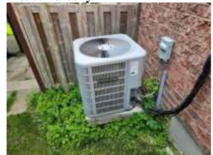
Pic. 9: AC unit 2012
