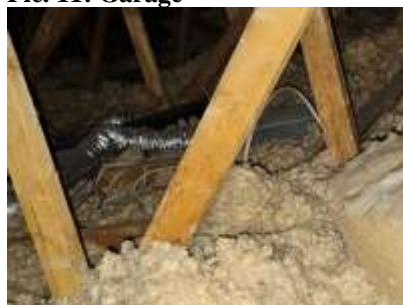
Pic. 14: 2 nd floor bathroom exhaust fan vent pipes tied together
