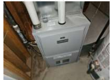
Pic. 45: Gas furnace 2017
