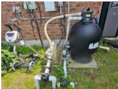
Pic. 7: Pool pump and filter
