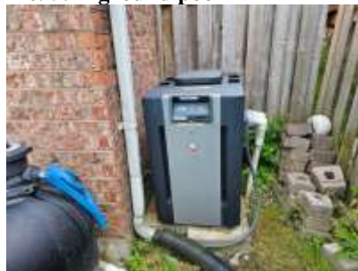
Pic. 8: Pool heater
