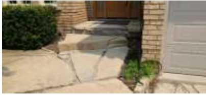
Pic. 4: Front steps with an uneven rise
