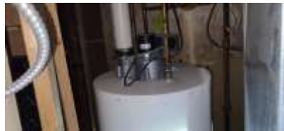
Pic. 35: Rental hot water tank
