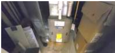
Pic. 34: Gas furnace 2018
