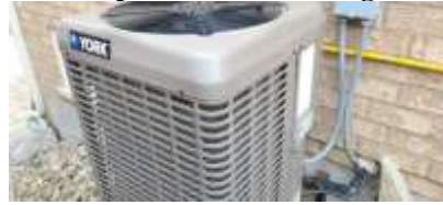
Pic. 5: AC unit 2018
