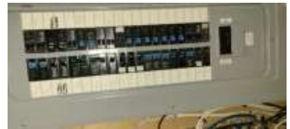
Pic. 36: 200 amp breaker panel
