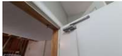
Pic. 11: Auto closer disconnected
