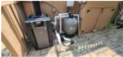
Pic. 7: Pool pump / heater / filter
