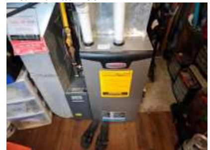
Pic. 30: New gas furnace
