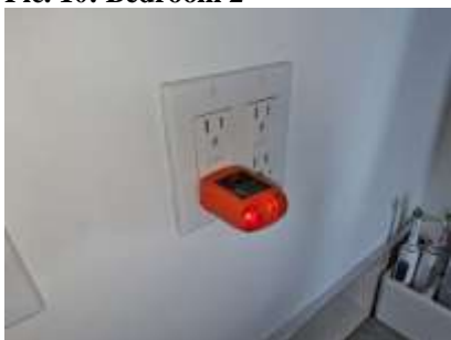
Pic. 13: GFCI outlets wired incorrectly
