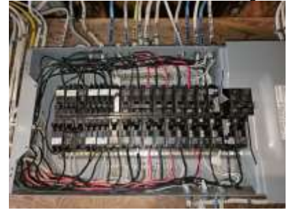
Pic. 33: Updated 100 amp breaker panel
