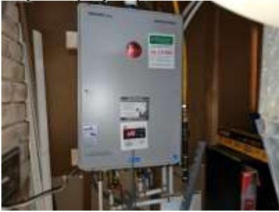
Pic. 31: Newer tankless hot water system
