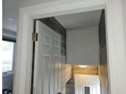
Pic. 20: Basement entrance door has the wrong swing – trip hazard
