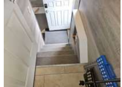
Pic. 21: Handrailing advised for upper section of basement stairwell
