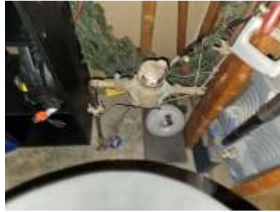
Pic. 32: Water main system
