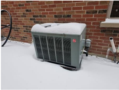
Pic. 4: AC compressor 2009
