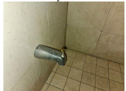
Pic. 15: Shower water diverter seized
