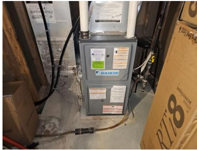
Pic. 38: Gas furnace 2016
