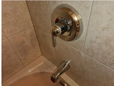
Pic. 20: Faucet drips of turned on – not tested
