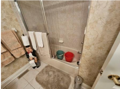
Pic. 19: 2 nd floor bathroom
