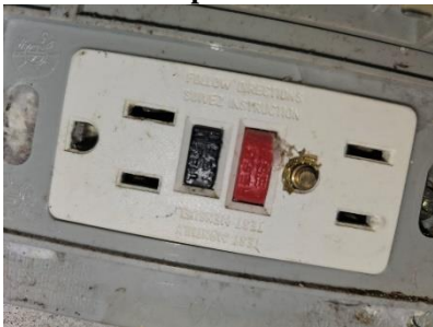
Pic. 7: Ground pin stuck inside exterior outlet needs to be removed
