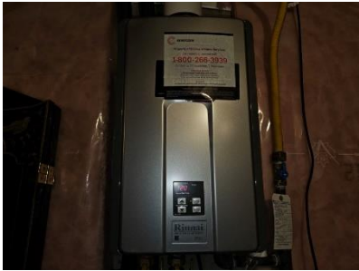
Pic. 37: Tankless hot water boiler 2011
