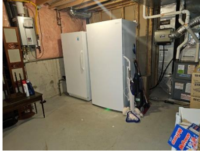
Pic. 35: Utility room
