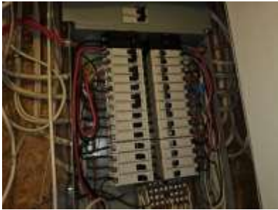
Pic. 52: 100 amp breaker panel
