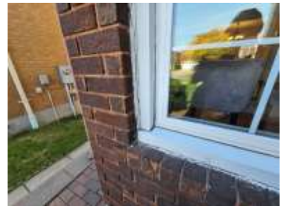
Pic. 12: regular caulking maintenance needed
