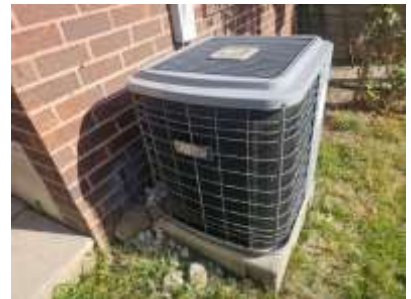
Pic. 9: AC compressor 2002
