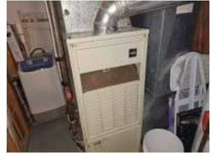
Pic. 51: Original gas furnace
