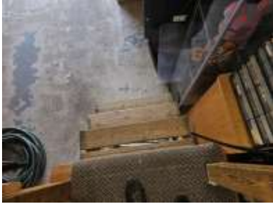
Pic. 16: Improper steps in garage
