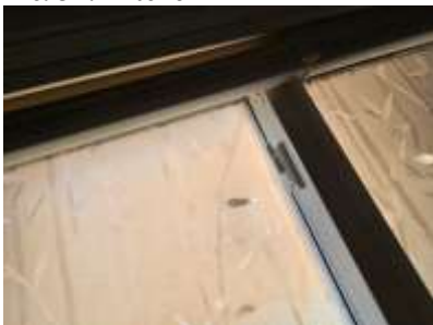
Pic. 37: Cracked window panel in office
