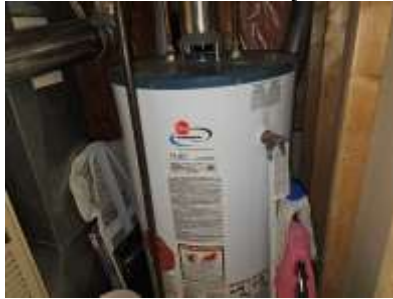
Pic. 50: Rental hot water tank 2009
