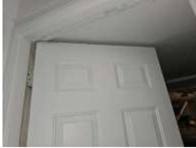
Pic. 17: No auto closer on garage entry door
