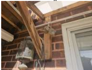
Pic. 8: Improper wiring on exterior
