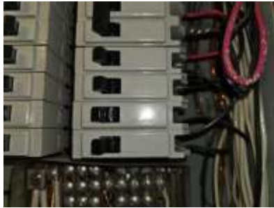
Pic. 53: A couple of breakers are double tapped
