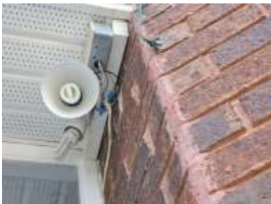
Pic. 13: Improper wiring at the front light fixture
