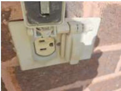
Pic. 10: No power at outlet
