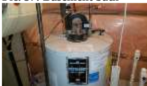
Pic. 41: Rental hot water tank
