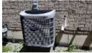
Pic. 3: AC unit 2007
