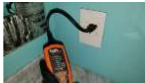
Pic. 15: GFCI not wired correctly
