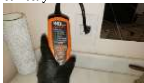
Pic. 19: GFCI not wired correctly
