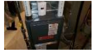
Pic. 40: Gas furnace 2014
