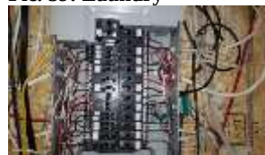
Pic. 43: 100 amp breaker panel
