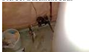
Pic. 42: Water main tank
