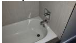
Pic. 23: 2nd floor bath
