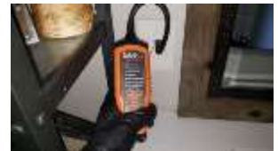
Pic. 24: GFCI not wired correctly
