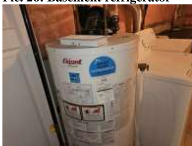
Pic. 29: Hot water tank 2017
