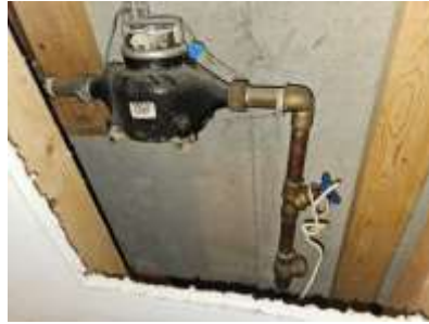
Pic. 32: Water main
