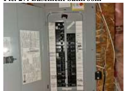
Pic. 30: 100 amp breaker panel
