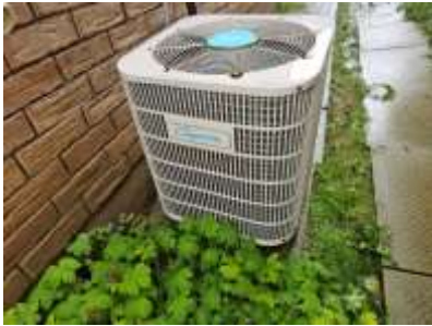
Pic. 4: Original AC unit
