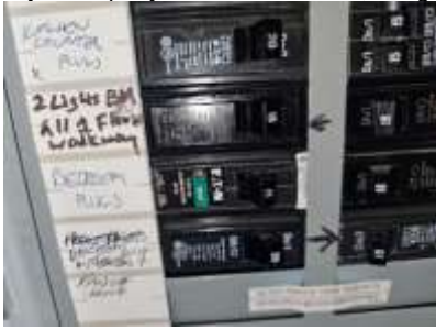
Pic. 31: ARCF breaker is defective and needs to be replaced
