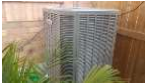
Pic. 5: AC unit
