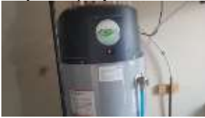
Pic. 25: Rental hot water tank
