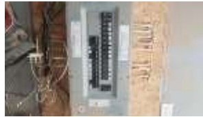
Pic. 7: 100 amp breaker panel with all copper wire
