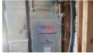
Pic. 26: High efficiency hot water forced air system
