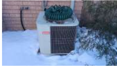
Pic. 5: AC unit 2000
