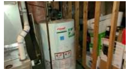
Pic. 30: Rental hot water tank
