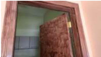
Pic. 7: No auto closer for garage entry door
