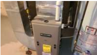
Pic. 31: Gas furnace 2017
