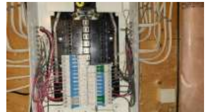
Pic. 33: 100 amp breaker panel
