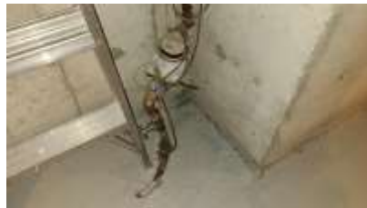
Pic. 32: Water main
