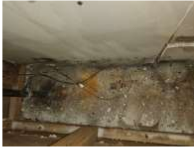
Pic. 35: Apparent visible mould in water meter cabinet, clean accordingly
