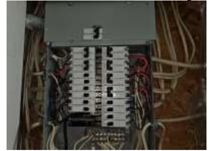
Pic. 33: 100 amp breaker panel
