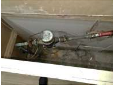
Pic. 34: Water main
