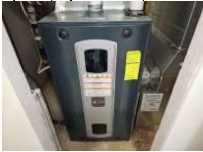
Pic. 31: Gas furnace 2018
