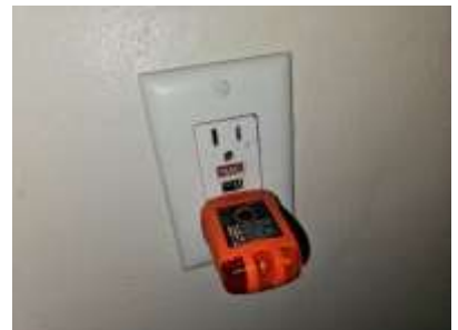
Pic. 30: GFCI outlet needs to be replaced
