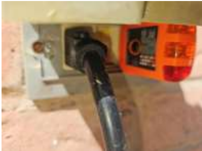
Pic. 7: Rear GFCI outlet needs to be replaced
