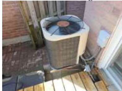
Pic. 8: AC compressor 2009
