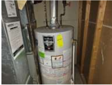
Pic. 32: Hot water tank 2012
