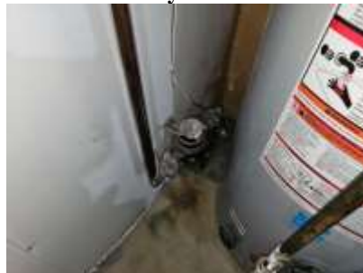
Pic. 38: Water main
