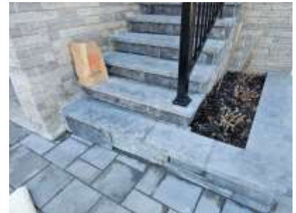
Pic. 9: Front steps uneven rise – first step too high Attic
