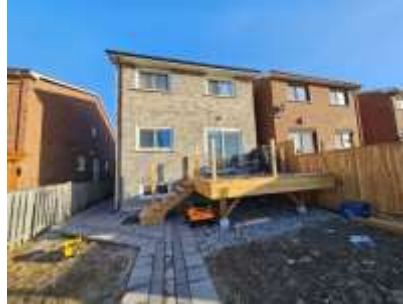
Pic. 5: Back view – railings needed for deck
