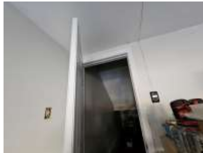
Pic. 8: Auto closer needed for garage entry door
