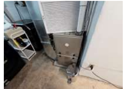
Pic. 36: Newer gas furnace
