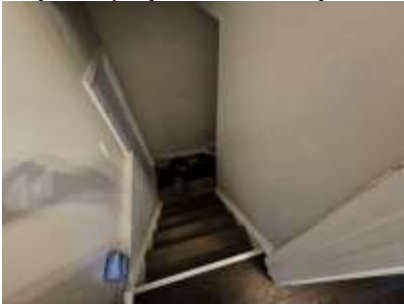
Pic. 28: Handrail needed for basement stairwell
