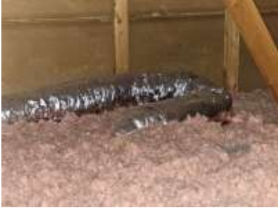
Pic. 13: Primary bathroom vent pipe not venting to the outside
