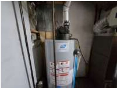
Pic. 37: Hot water tank
