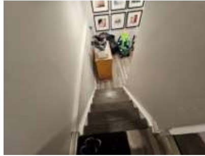
Pic. 29: Handrail needed for basement stairwell
