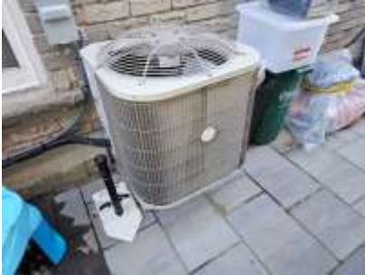
Pic. 4: Newer AC compressor
