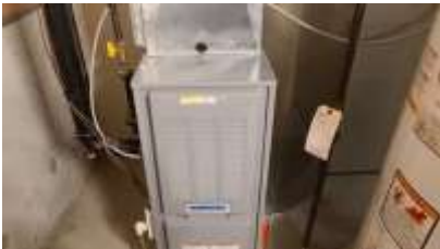
Pic. 25: Original gas furnace 2002
