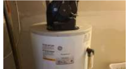
Pic. 24: Hot water tank
