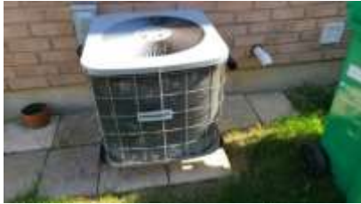
Pic. 4: AC unit 2001
