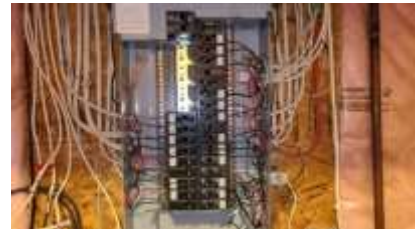
Pic. 27: 100 amp breaker panel
