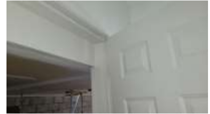
Pic. 6: Auto closer needed for garage entry door
