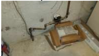
Pic. 26: Water main
