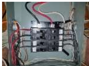
Pic. 38: Sub panel – one breaker double tapped
