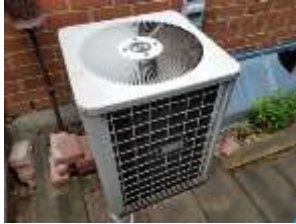
Pic. 5: AC unit – 1999
