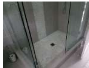
Pic. 15: 2 nd floor bath
