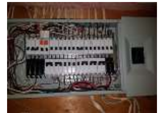
Pic. 36: 200 amp breaker panel with all copper wire
