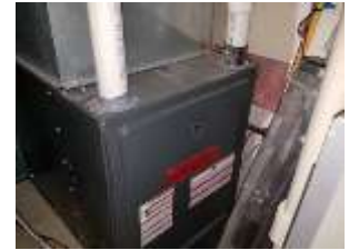
Pic. 32: High efficiency gas furnace 2012
