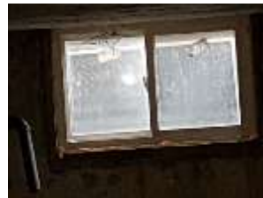
Pic. 35: Window cracked
