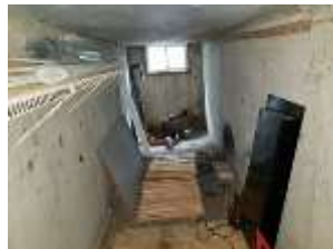
Pic. 34: Cold room
