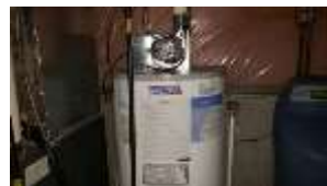
Pic. 27: Rental hot water tank
