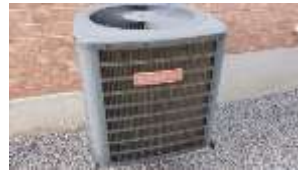
Pic. 3: AC unit 2009
