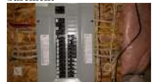
Pic. 28: 100 amp breaker panel
