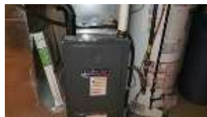
Pic. 26: Original gas furnace
