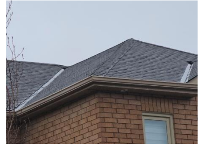
Pic. 3: Roof covering – showing some age
