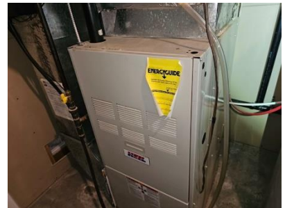
Pic. 39: Gas furnace 2000
