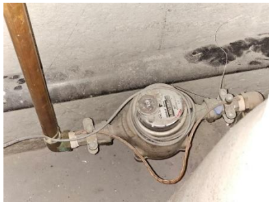
Pic. 41: Water meter
