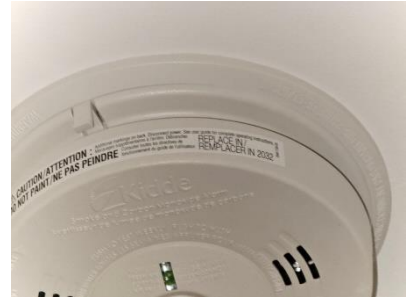
Pic. 21: Smoke detector expire 2032
