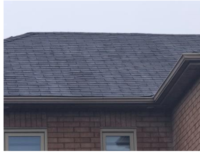
Pic. 2: Roof covering – showing some age
