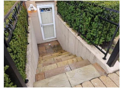
Pic. 6: Handrailing advised for exterior stairwell
