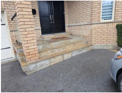
Pic. 4: Uneven rise on front steps
