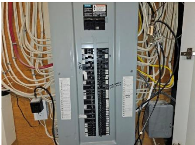
Pic. 40: 200 amp breaker panel
