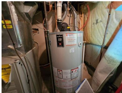
Pic. 38: Water heater 2012
