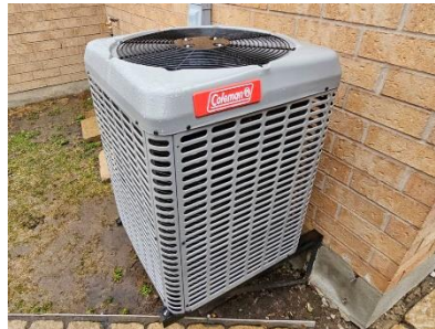
Pic. 8: AC unit 2020
