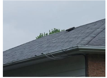
Pic. 3: Aging roof covering
