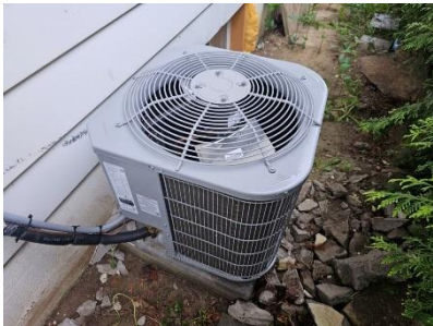
Pic. 7: AC unit 2023
