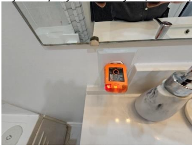
Pic. 16: Bathroom outlet wired incorrectly and not GFCI protected
