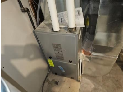
Pic. 31: Gas furnace 2023
