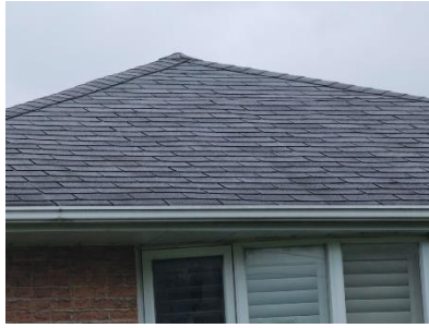
Pic. 2: Aging roof covering
