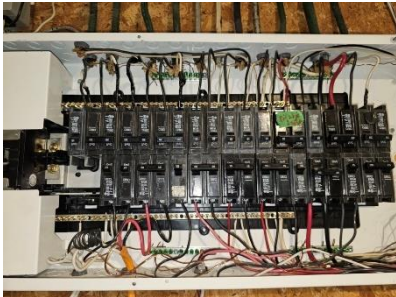
Pic. 34: All copper wiring
