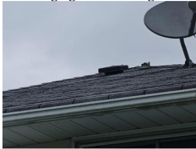
Pic. 5: Aging roof covering
