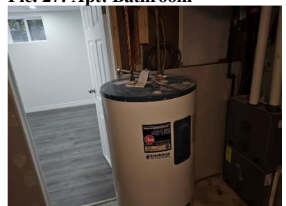
Pic. 30: Electric hot water tank 2008
