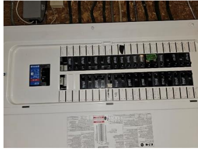
Pic. 32: 200 amp electrical panel – opening at front of the panel need to be sealed
