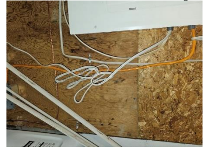
Pic. 33: Wires need to be properly secured
