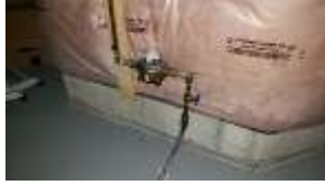
Pic. 29: Water main
