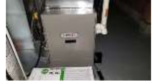
Pic. 31: Gas furnace
