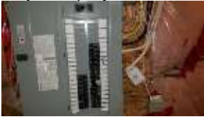
Pic. 32: 200 amp breaker panel
