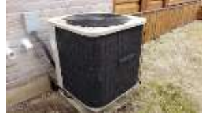
Pic. 3: AC unit
