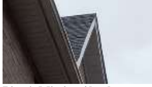
Pic. 6: Missing / broken shingle tabs on rear roof
