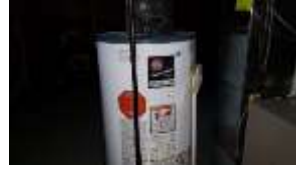
Pic. 30: Rental water heater
