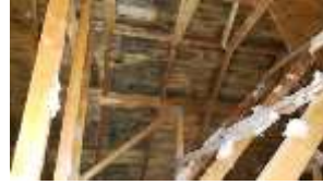
Pic. 7: Some moderate apparent mould growth present – See Attic Comments
