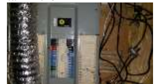
Pic. 28: 100 amp breaker panel
