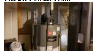
Pic. 24: Rental hot water tank 2013
