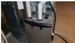
Pic. 25: Gas furnace 2014
