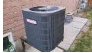
Pic. 3: AC unit 2005
