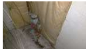
Pic. 27: Water main
