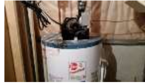
Pic. 27: Rental hot water tank – 2000
