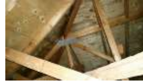
Pic. 7: Minor staining on sheathing over master bath
