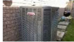
Pic. 3: AC unit – 2015
