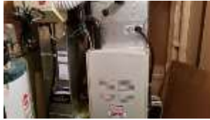
Pic. 26: High efficiency gas furnace - 2000
