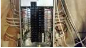
Pic. 29: 100 amp breaker panel with all copper wire
