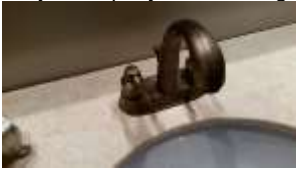
Pic. 25: Hot water faucet need repair / replacement
