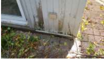
Pic. 4: Wood siding with some rot at the bottom
