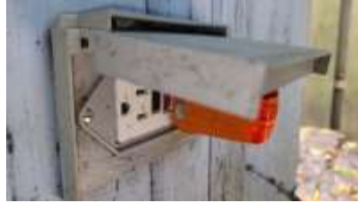
Pic. 5: Rear GFCI outlet defective and needs to be replaced
