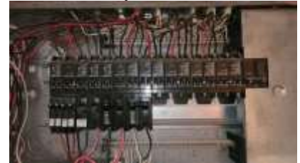
Pic. 24: 100 amp breaker panel
