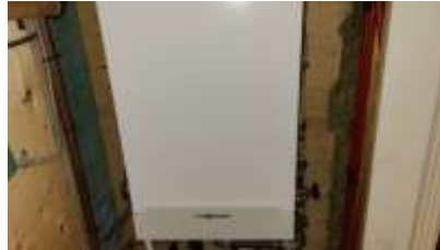
Pic. 23: Tankless hot water / boiler system
