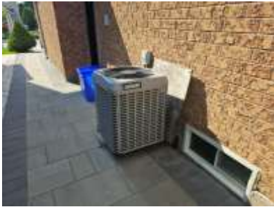
Pic. 4: AC compressor 2018
