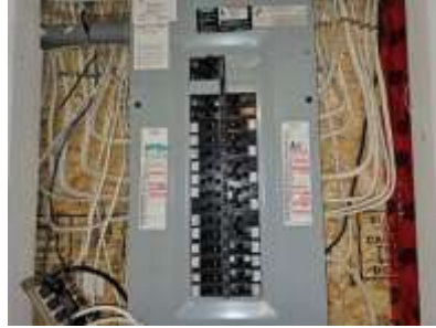
Pic. 35: 100 amp breaker panel
