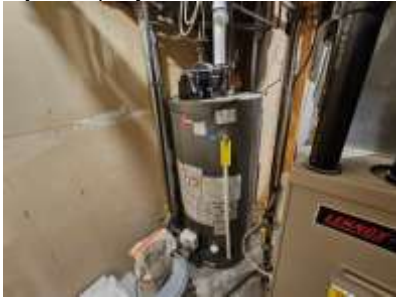
Pic. 31: Rental hot water tank 2019
