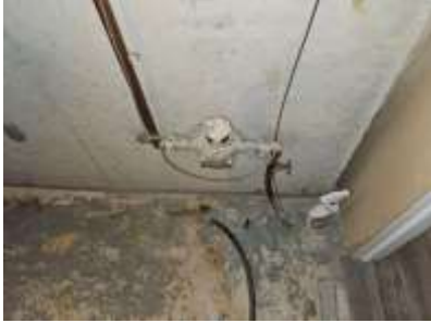
Pic. 34: Water main
