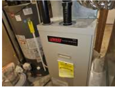
Pic. 32: Original gas furnace
