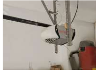
Pic. 6: East garage door opener not working
