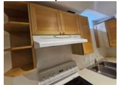
Pic. 27: Exhaust fan not working
